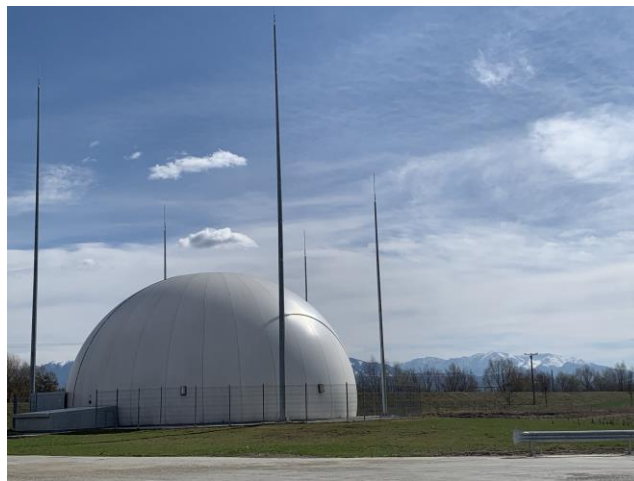
Fig .5 -Unitate de stocare biogaz GH820
