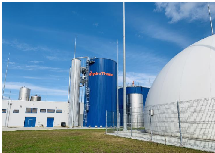
Fig. 3 – Reactor ECSB (HydroThane)
