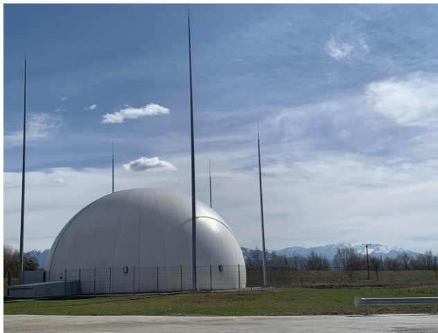
Fig .5 -Unitate de stocare biogaz GH820
